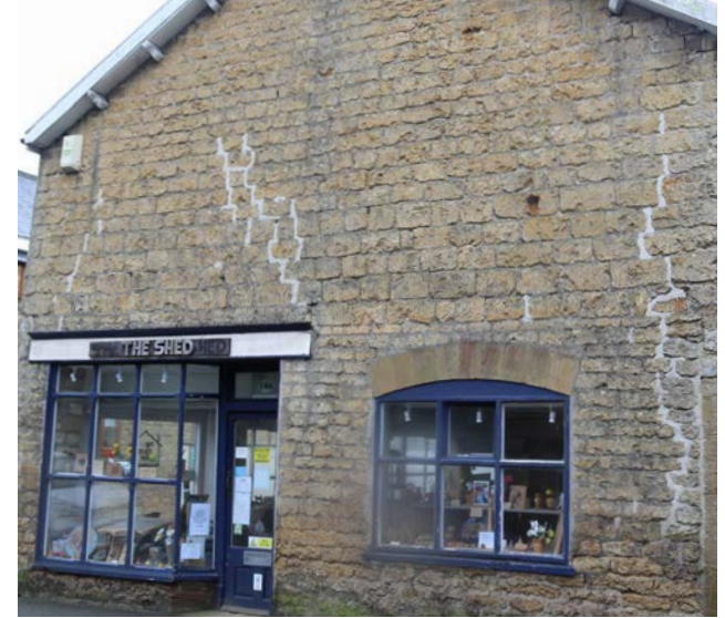
Figure 11: Example of repointed sections in sand and cement mortar beside traditional lime mortar.
